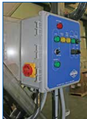
System control panel includes lockout, 24 volt transformer and waterproof switches & illuminated indicator lights for improved safety and automatic or manual operation.
