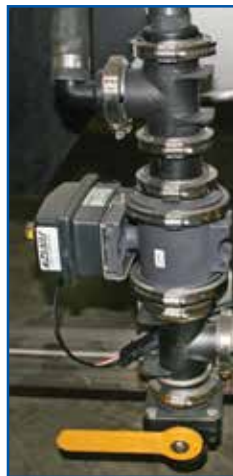
Large 2" water inlet plumbing includes 24 volt automatic control valve, manual throttling valve & drain valve. Overflow protection also included.
